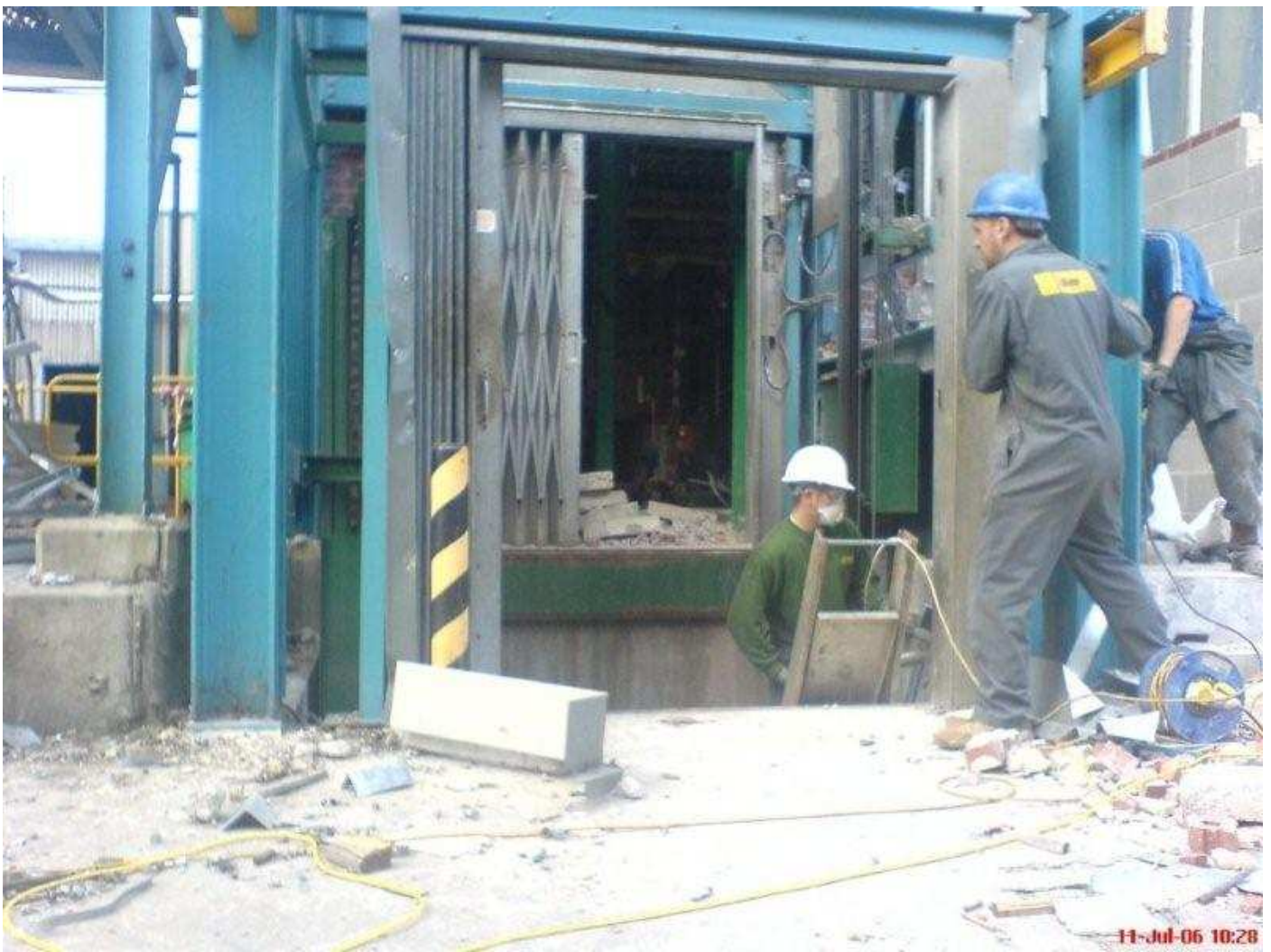
Above – Preparing the entry and exit points so the lift was free for removal.
