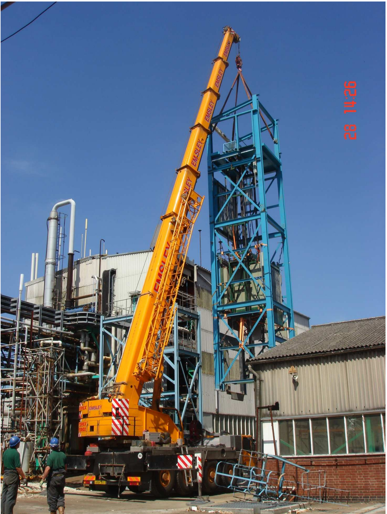
Above – Some careful calculations were made beforehand to ensure the right size of crane was used as no weights were available from the manufacturers. The bespoke lifting points and bracing used were designed by our engineers specifically for this job. As a side note we couldn't have asked for better weather.
